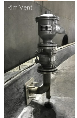
Vacuum Breaker / Bleeder Valve
